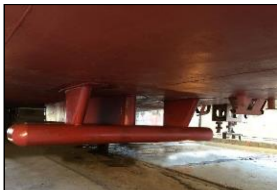
The 7150F echosounder multibeam installed.
